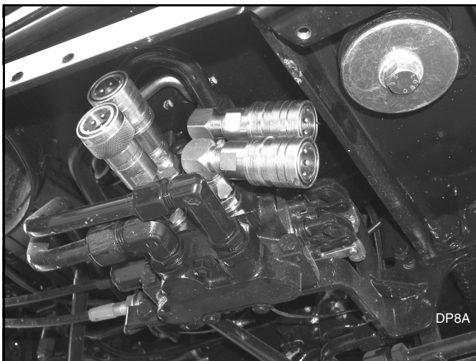
Figure 11. Hydraulic Fitting Installed, Bottom View
